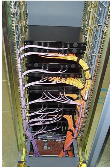
Figure 7 – Cable management in racks
